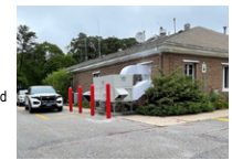
Interim HVAC improvements located to minimize sound issues and structure modifications
